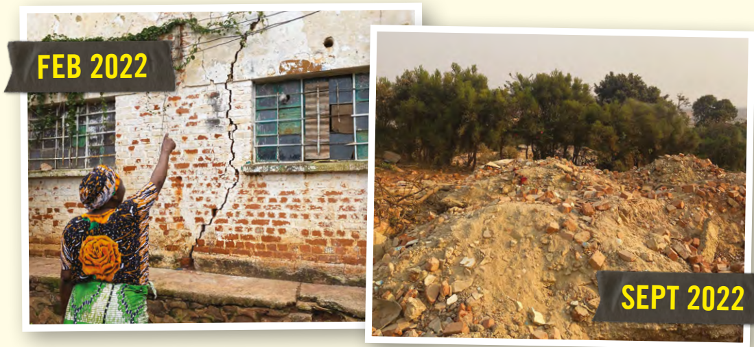
© ↑ Cécile Isaka showing crack in her house caused by the activities of the Kolwezi copper and cobalt mine operated by COMMUS, February 2022 (left); Ruins of Cécile Isaka’s house, September 2022 (right) © Amnesty International (photographer: Jean-Mobert Senga)
